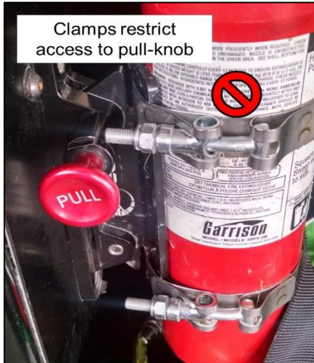
Image B-44.2: Fire Extinguisher, Incorrect orientation of extinguisher clamps
